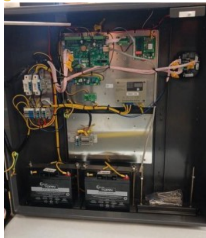
Sign Activated via Local Controller
