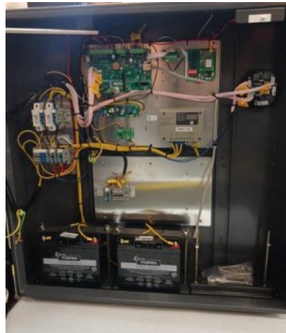
Sign Activated via Local Controller
