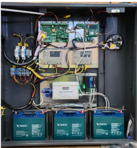
Sign Activated via SmartSign
