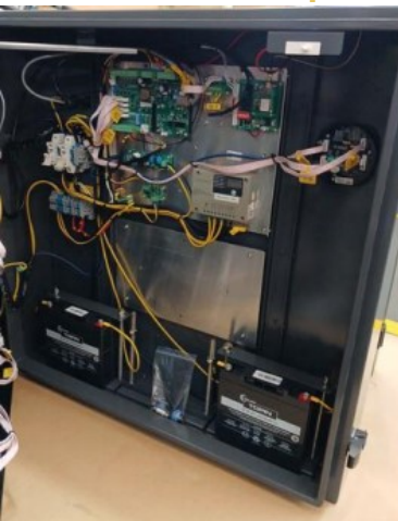
Sign Activated via SmartSign
